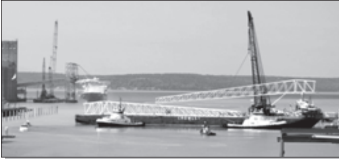
Above, A 450 ton barge crane getting ready to erect a cantilever truss section. Right, 230 foot truss sections going up.
